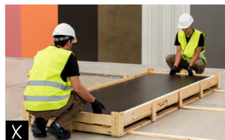
✗ Do not position yourself opposite your workmate to remove the ceramic slabs from the box.
