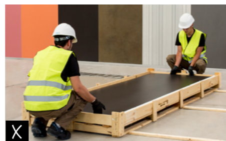
✗ Do not position yourself opposite your workmate to remove the ceramic slabs from the box.
