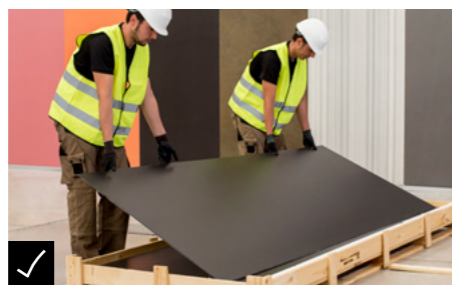
✓ Hold the ceramic slab with both hands and raise it slowly. Do this at the same time as your workmate.
